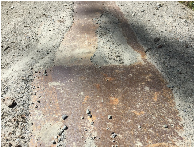
Minor deck deformation noted on wheel path
